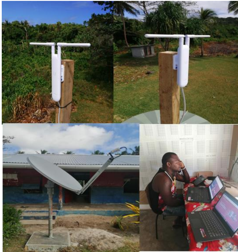
Installation by Vodafone on Toka Island, Torba Province
