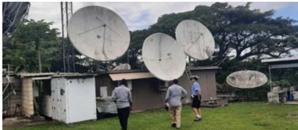
Equipment inspection of Telsat Pacific equipment
